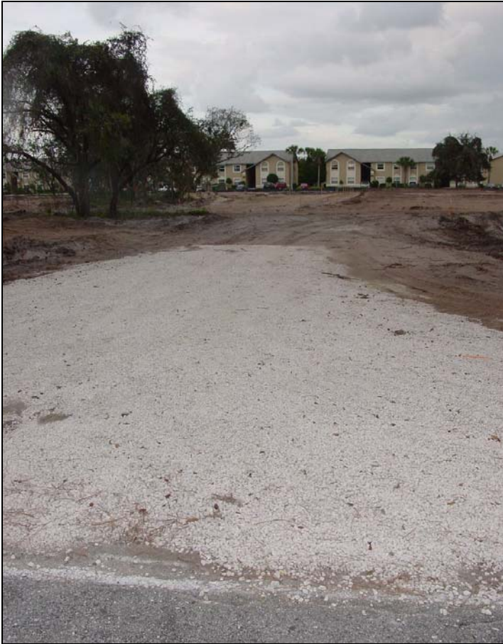
A stone stabilized pad located at points of vehicular ingress and egress on construction sites reduce the amount of sediment transported to public roads by motor vehicles or runoff.
